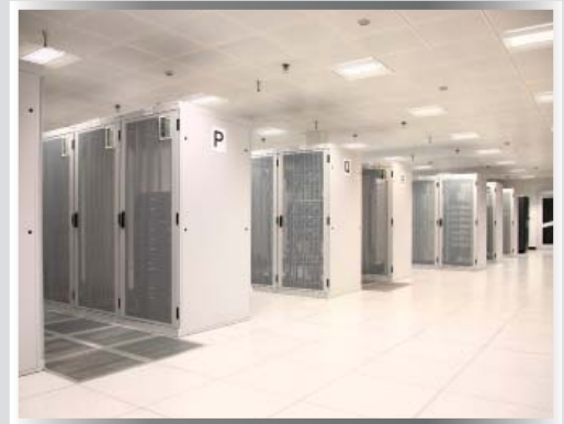
Data center, including control room, tape room and three battery rooms
