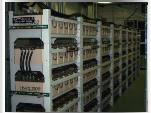
A data center in the Midwestern United States is using VESDA ECO for hydrogen detection in three battery rooms.
